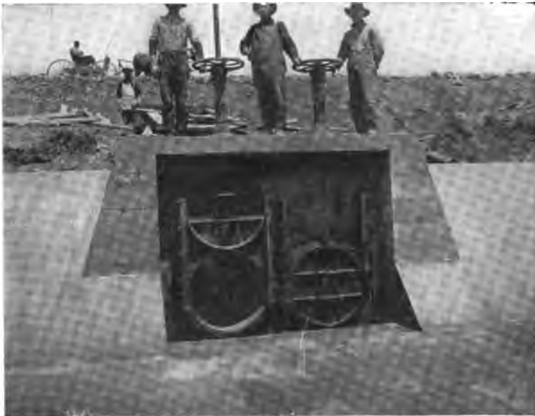
FIG. 105.—Cast-iron Valve on Small Lateral Turnout.
